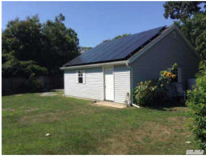
Solar Panels Provide Electric to Home
